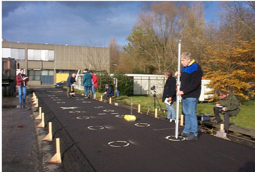
Figure 5.4 All measurements (temperature, level and rod, Strato test and Troxler) in progress and an illustration of measuring point indicators.
